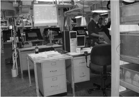
The engine room is monitored remotely. (Photo: R.H. Wagner).
