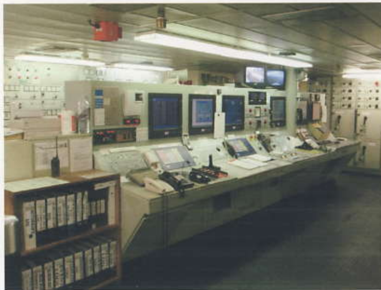
ARTEMIS Engine Control Room
